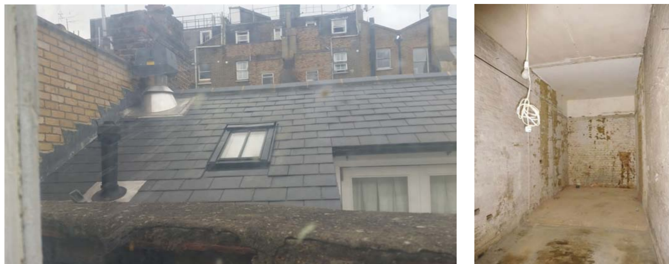
Fig 3 View from rear window towards 57 Lancaster Mews and internal ground floor space
